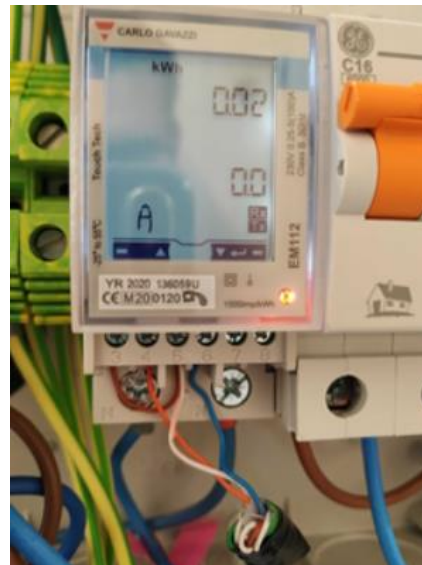
Good installation of meter connections (note RXTX and bridge)
