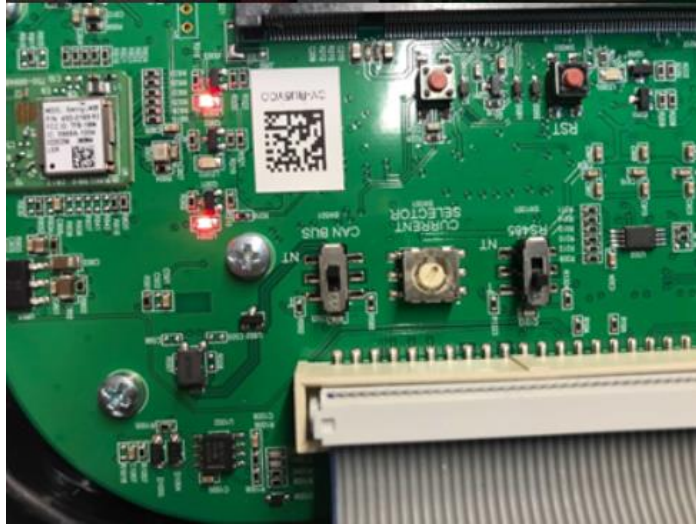
Close up CAN bus switches
