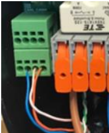
Good installation of modbus on HV-side
